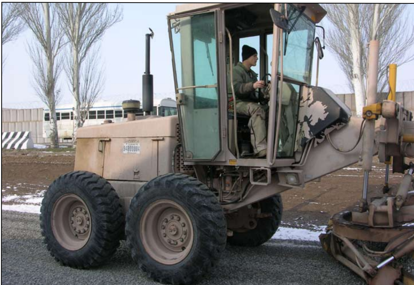
Airman 1st Class Joshua Colwell, 376th Expeditionary Civil Engineer Squadron "Dirt Boyz" grades gravel at Manas Air Base. Airman Colwell is one of an eight-person crew dedicated to most construction and repair projects here. (Air Force photos by Master Sgt. Tonie Atkinson)
